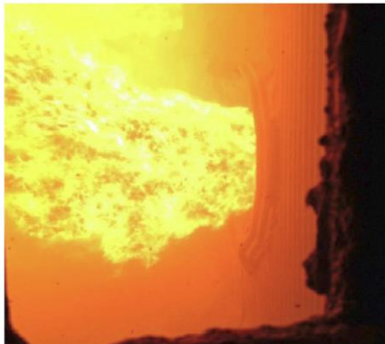
Figure 1: Burner flame in a coal fired power plant
